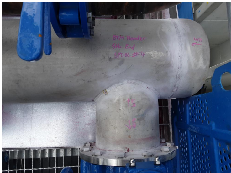
Image 1 of 6 - Bottom header South end spool #4 W9-11
