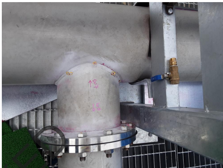
Image 2 of 6 - Bottom header South end spool #4 W7-8
