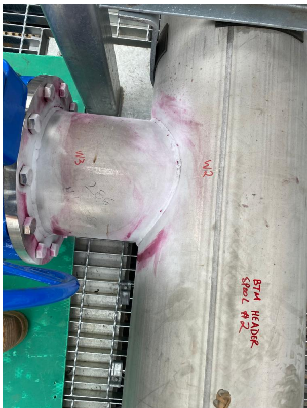
Image 5 of 13 - Bottom header spool 2 W2 & W3
