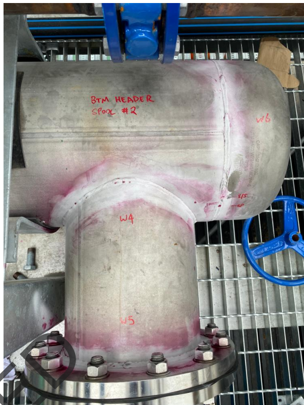
Image 10 of 13 - Bottom header spool 2 W4, W5 & W6
